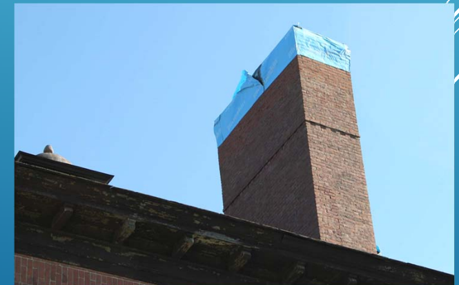
Chimney Wrap Failing
