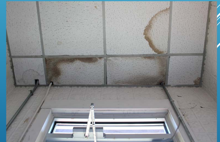
Leaks At Side Entrance Vestibule
