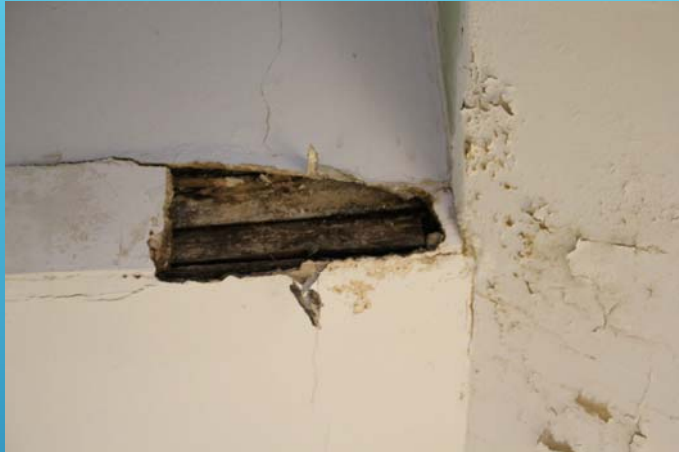
Leaks Causing Falling Plaster
