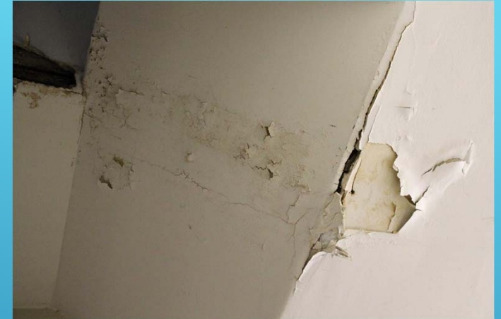
Leaks Causing Peeling Paint
