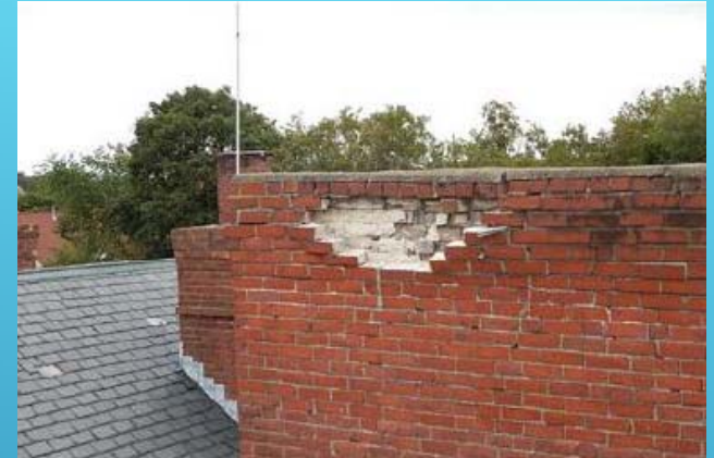
Brick Veneer Failing
