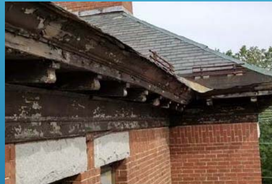
Damaged Ice & Snow Guards
