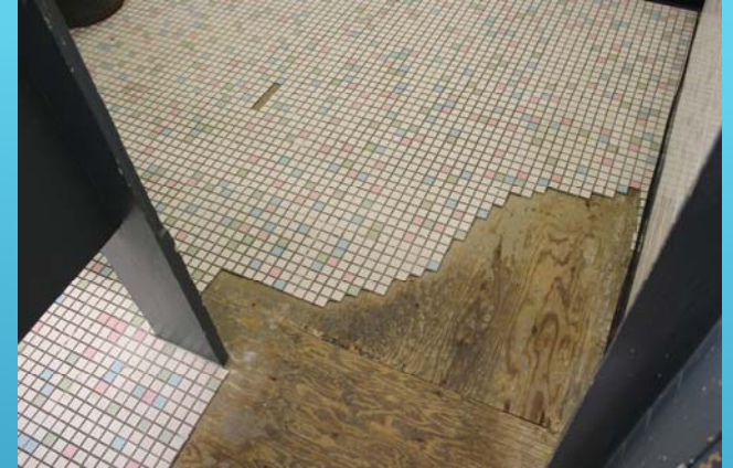
Missing Tiles - Inadequate substrate
