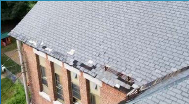
Falling Slate Roof Tiles
