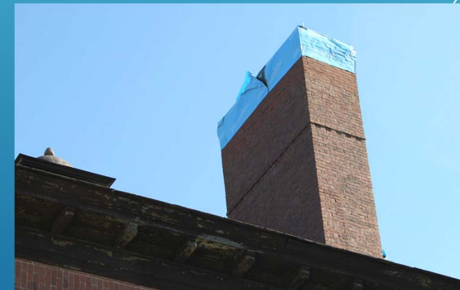
Chimney Wrap Failing
