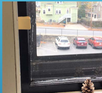
Rattling Drafting Windows
