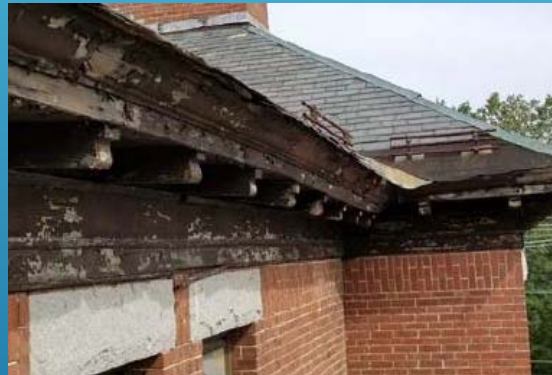
Damaged Ice & Snow Guards
