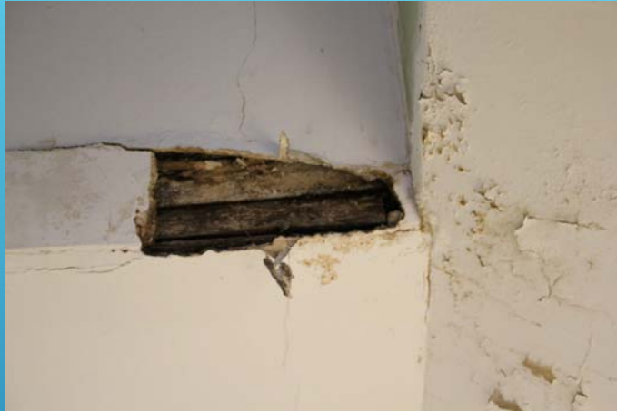
Leaks Causing Falling Plaster
