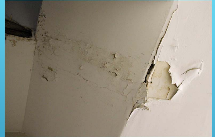
Leaks Causing Peeling Paint
