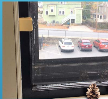
Rattling Drafting Windows
